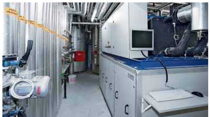
This waste water heat pump with 150 kW output is used for DHW heating.
