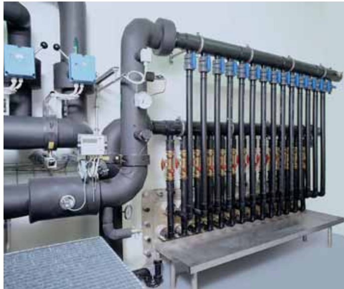
Geothermal probe manifold
