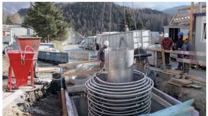
This waste water shaft is used as a primary source for DHW heating.
