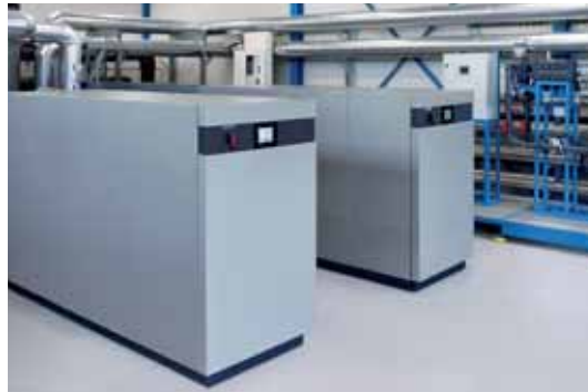
Vitocal 350-G PRO heat pumps with a total output of 620 kW
